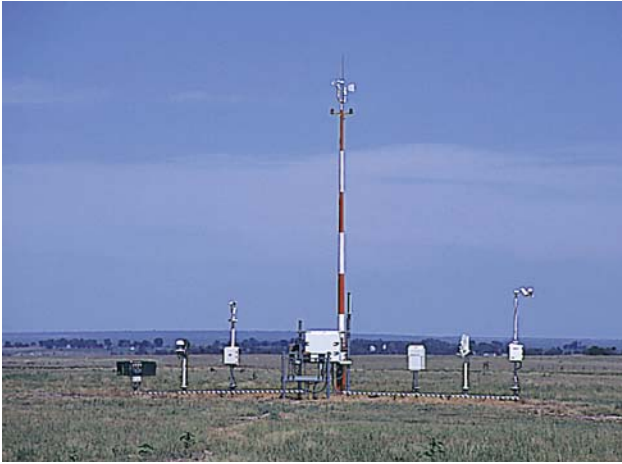
Figure 2-12. ASOS Station Installation.
