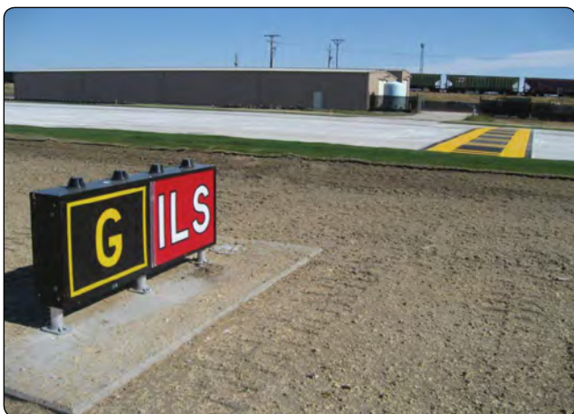
Figure 14-24. Instrument landing system (ILS) holding position sign and marking on Taxiway Golf.
