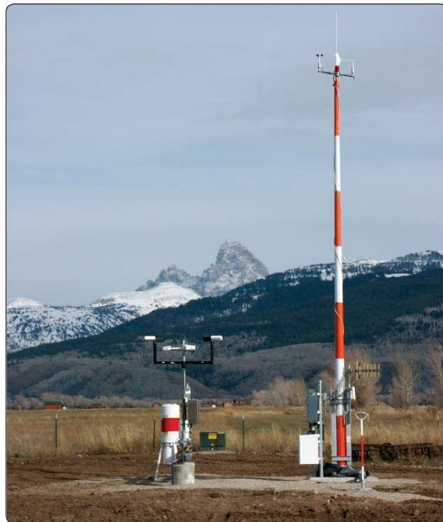
Figure 1-11. AWSS installation at Driggs-Reed, Idaho.
